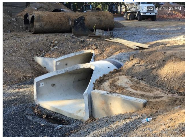
Storm drain piping at Beverly
